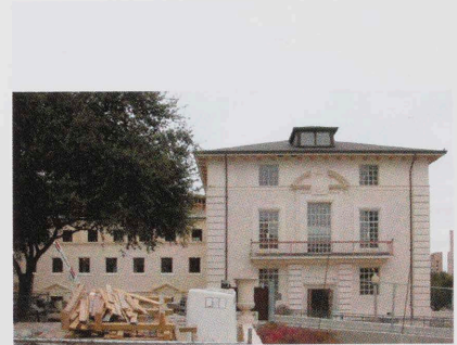
Benedict-Mezes connection, the most recent part of the sixpack, under construction in 2004
