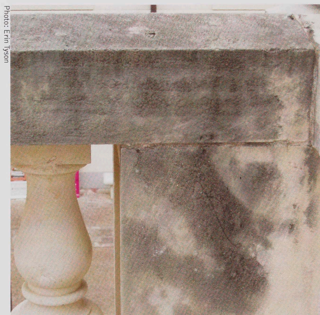
Biological staining on the east façade of Goldsmith Hall
