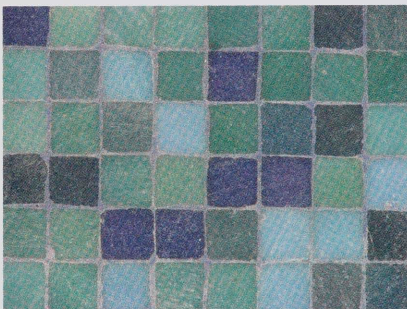
Glass mosaic tiles cladding the fourth floor loggia of the Flawn Academic Center
