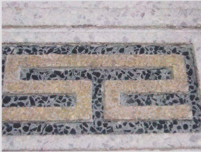
Earley Process Concrete on the walls of the first floor loggia of the south façade of the Main Building
