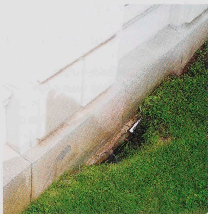
Landscape irrigation in use at the east side of Main Building is discharging excessive amounts of water against the building, causing long term damage to the foundation.
