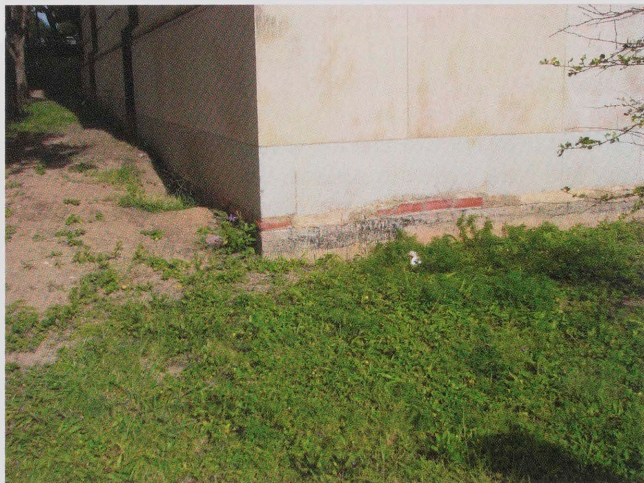
Soil erosion at grade outside Waggener Hall
