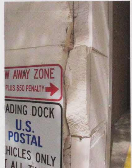
Mechanical damage at loading dock
