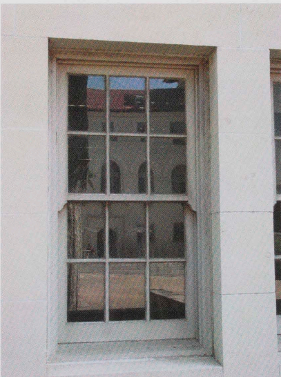
Wooden double hung window on Goldsmith Hall. All wooden windows of this type on campus feature decorative horns below the sash.
