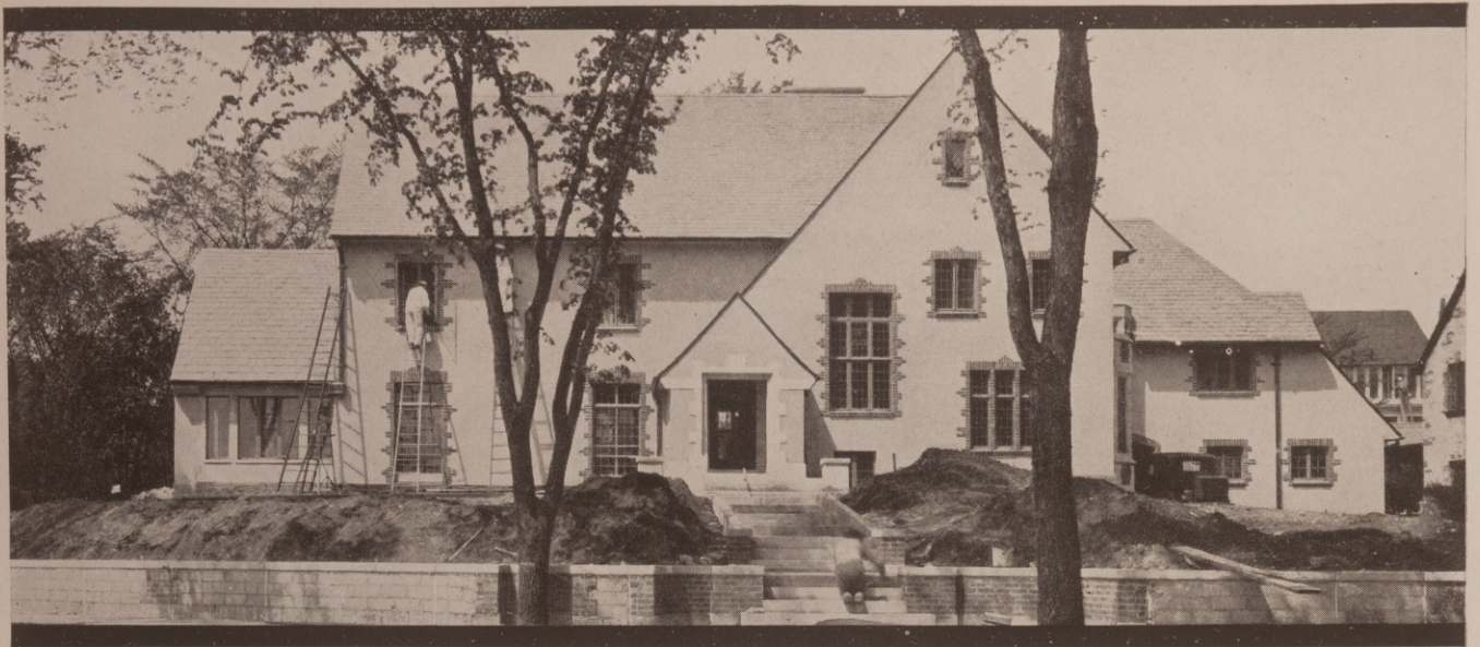
Provision is made for telephone convenience in the residence of Mr. J. R. Stewart, 2424 West Lake of the Isles Boulevard, Minneapolis, Minnesota, by built-in conduit serving six telephone outlets, including one in the basement game room. CARL A. GAGE, Architect, Minneapolis.
